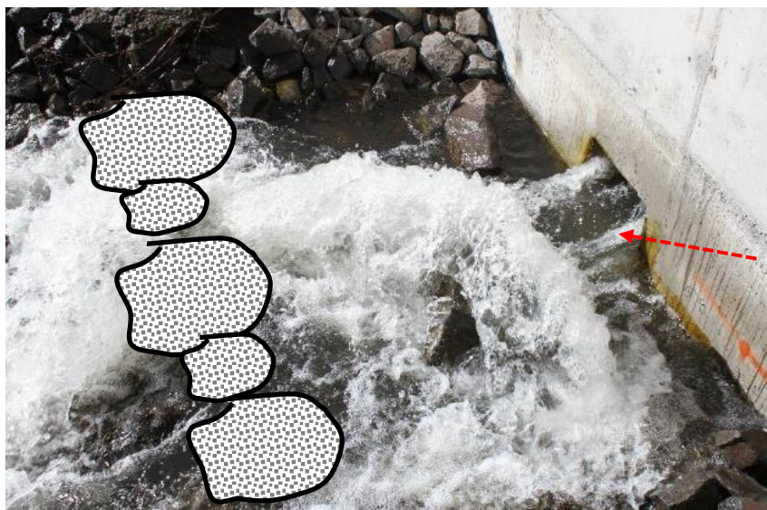
Figure 3.7: Upstream fish passage exit at Akhalkalaki 2 where flow speed (pressurised flow) combined with the thickness of the wall / opening may represent a barrier to upstream fish migration. Checks of passability should be undertaken and corrective measures implemented if needed, for instance placement of rocks to raise the water level immediately downstream of the opening.
