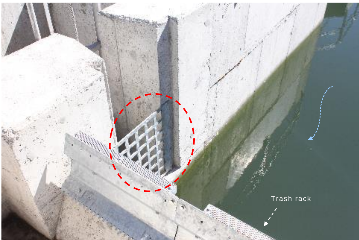
Figure 3.9: Entrance of the fish diverter (red ellipse) next to the trash rack at the sedimentation basin at Akhalkalaki 1 intended to safeguard downstream fish migration by minimising fish entering the waterway.
